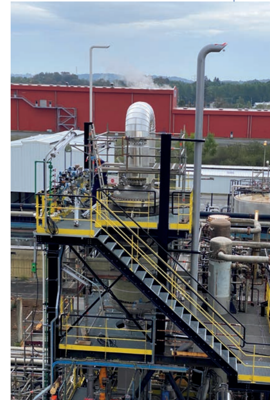
The new EkiNOx facility within the nitrosyl sulphate production unit.
