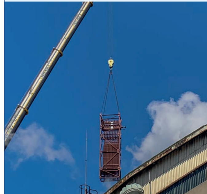
A crane installing the superheater boiler at the Marseille site through the roof of the boiler room
